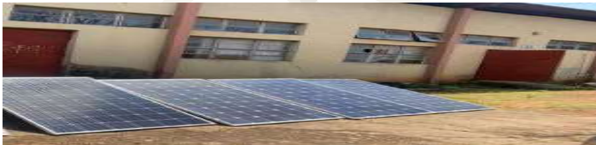
Figure 2: The solar panels
